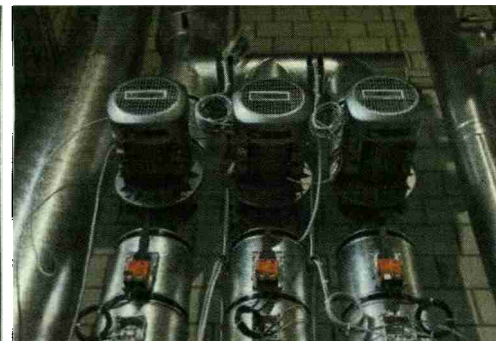
Pumpen speisen Warmwasser ins System.
